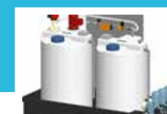
Sodium hydrogen carbonate dosing
